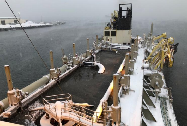
PHOTO 3: SECOND DREDGING SEASON; ON THE TRAILING SUCTION HOPPER DREDGERS (TSHD) WITH FULL HOPPER, READY TO SAIL TO DAS (DISPOSAL AT SEA) SITE (JANUARY 2020)
