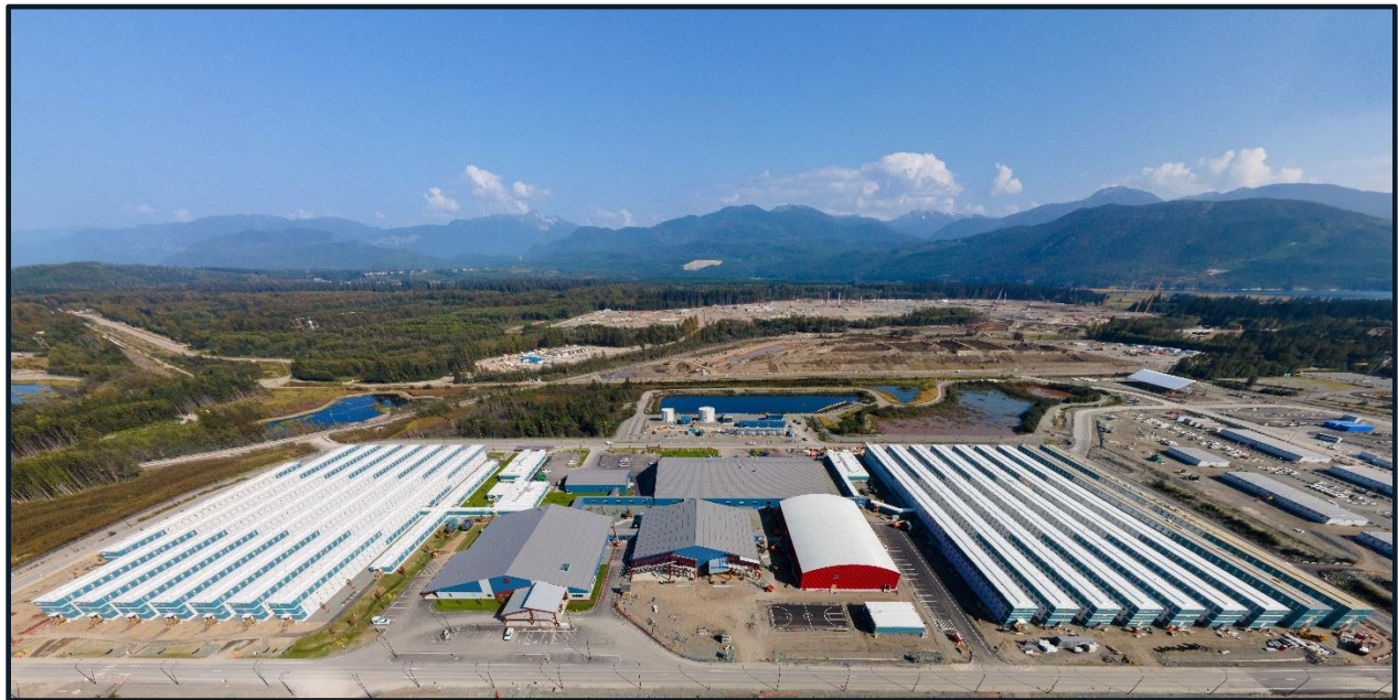
Figure 5 illustrate some of the Project construction activities that took place in 2020 Q3.
