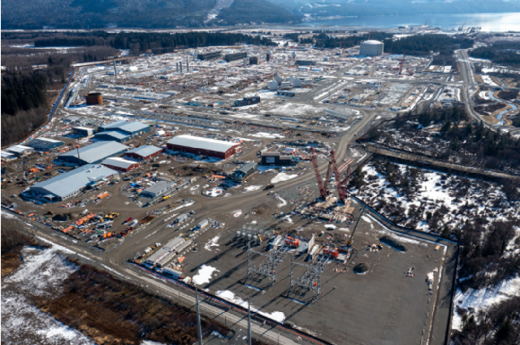
PHOTO 5: LNG FACILITY – DRONE SHOT (FEBRUARY 2022)
