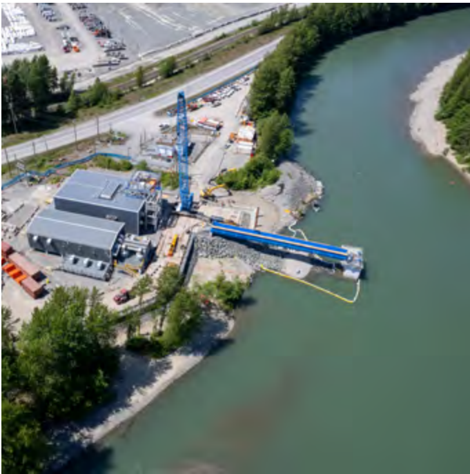
River water intake, where there are water inlet screens and a pump house to bring water from the Kitimat River to the LNG Canada site.
