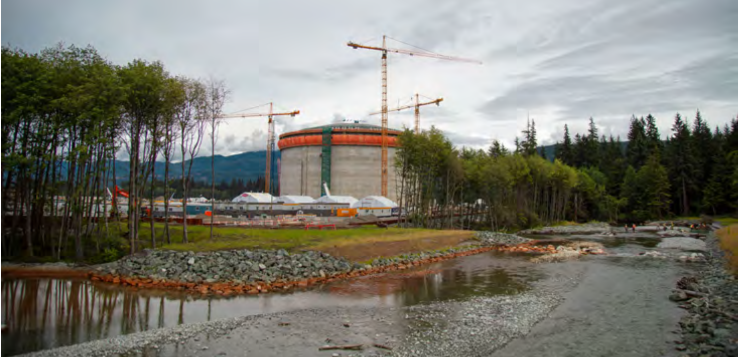
Anderson Creek Realignment fish habitat offset, located south of the LNG Canada plant site.
