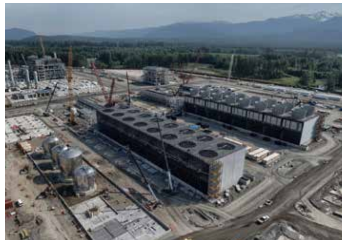
LNG infrastructure at main operations area
