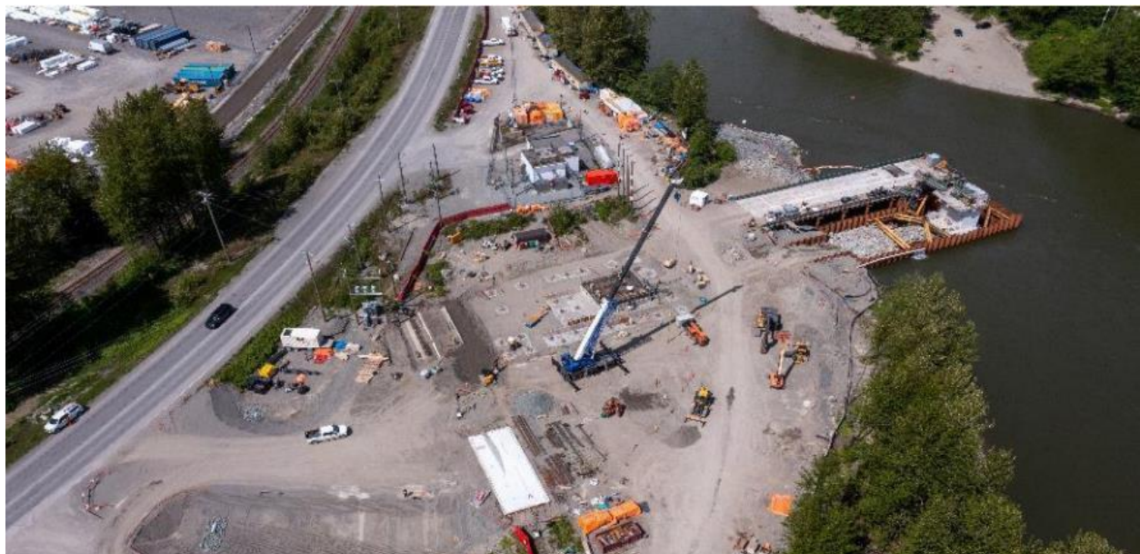
Figure 3 River Water Intake Pumpouse (2021 Q2)
